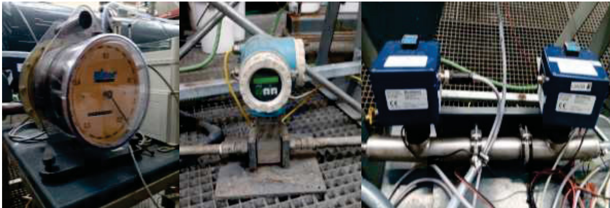
Figure 13 – Gas clock (left), flow meter (middle), gas analyzers (right)
