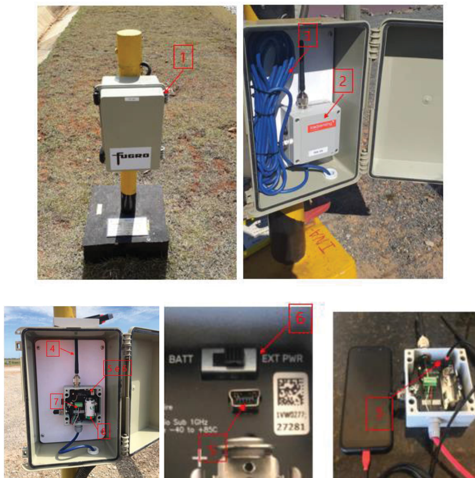
FIGURA 3.13 Datalogger local wireless
