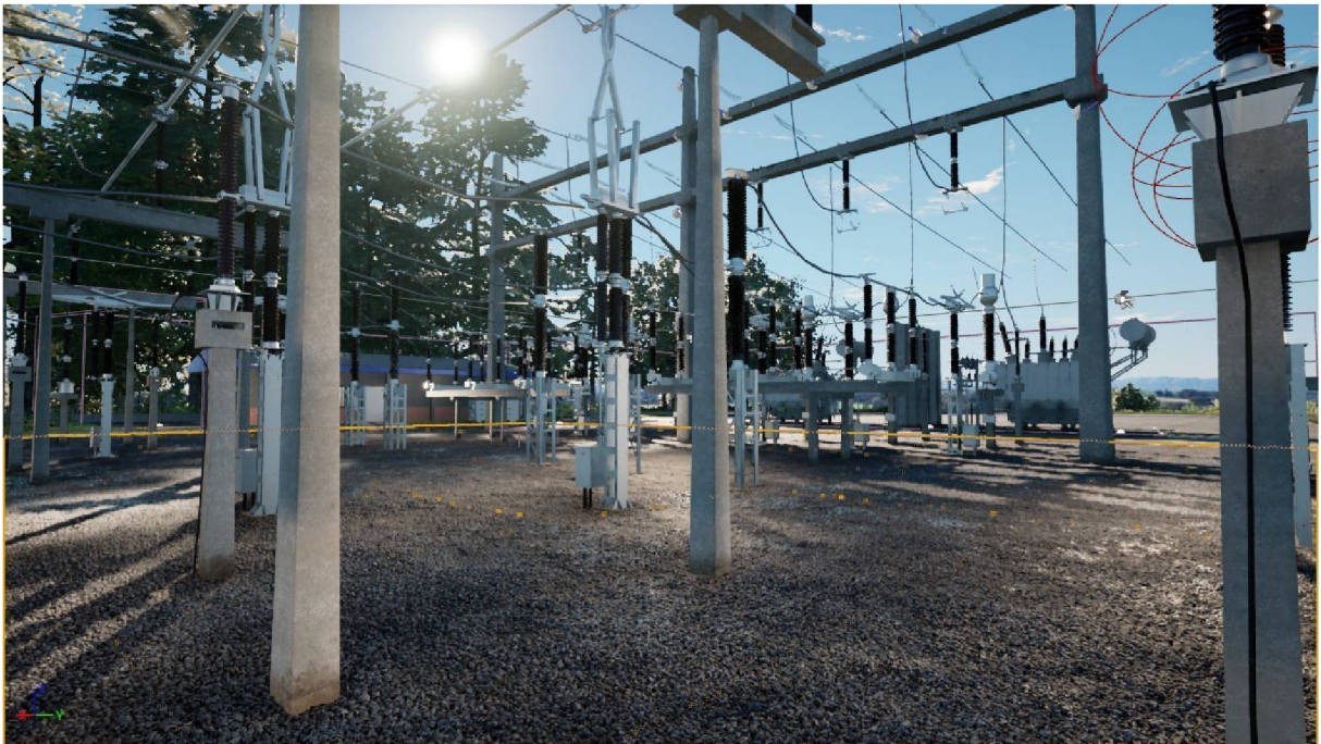
FIGURE 19 – A view of the equipments in the ground level. Source: OneReal research group.
