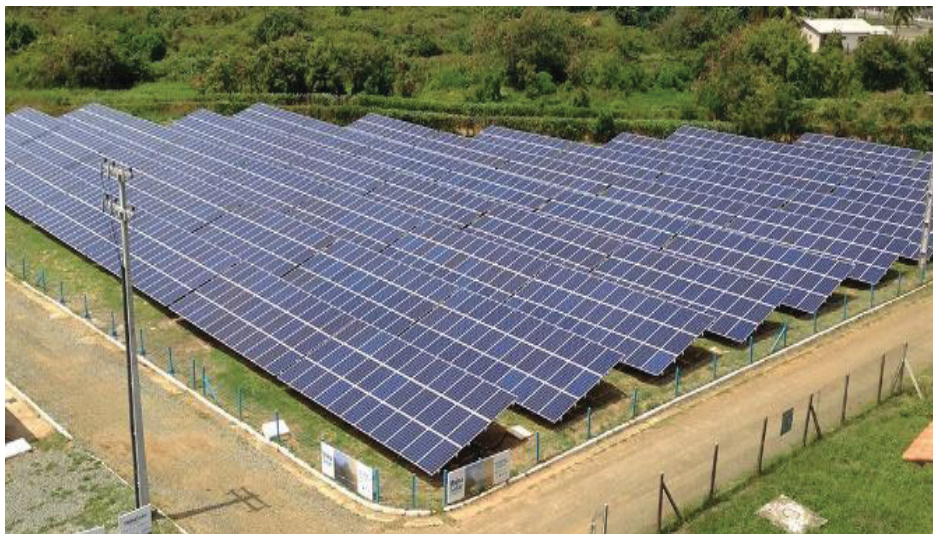
FIGURE 22 - NORONHA I SOLAR PLANT
