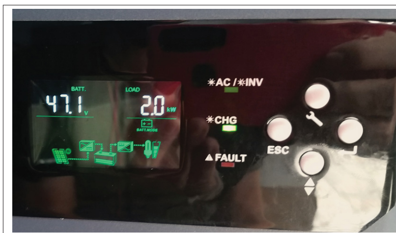
FIGURA 25 – Vista painel do inversor Off-Grid
