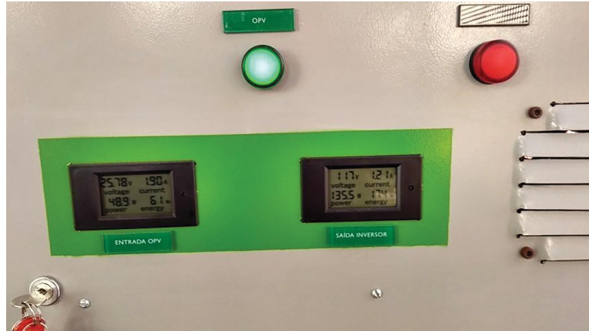
FIGURE 3.4: Front door of the distribution board. Green light on meaning the bus station is being powered by the OPV modules.
