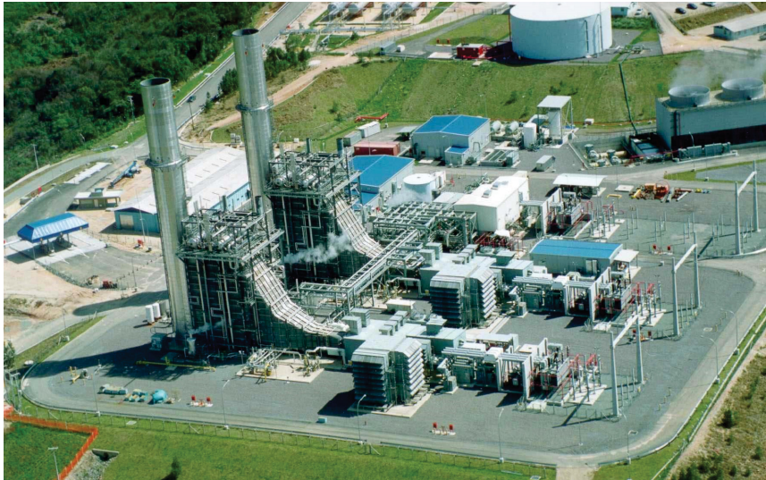
Figure 1.3: Exhaust towers view of the UEGA power plant at Araucária, Parana State, Brazil.
