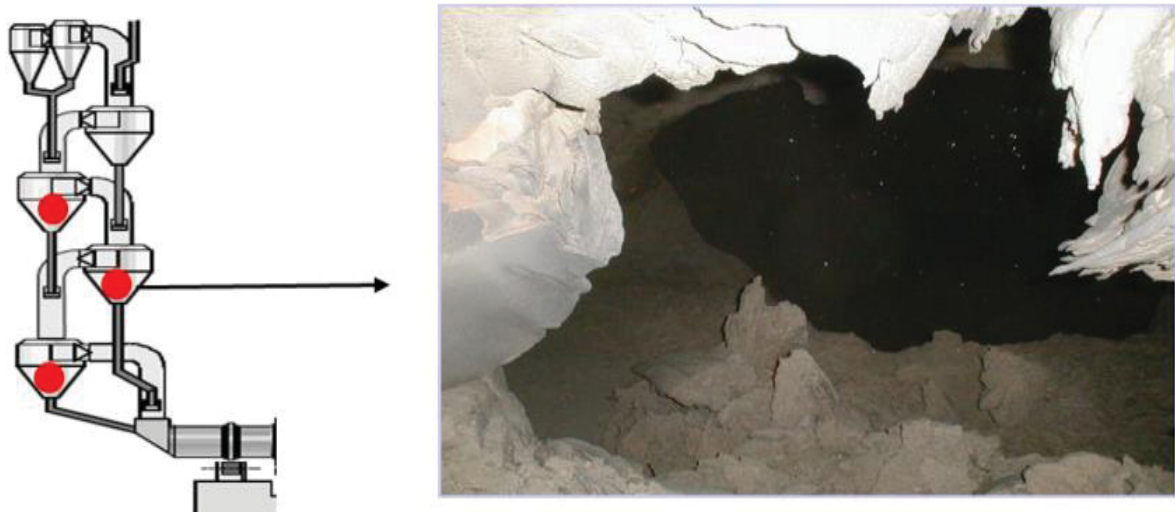
FIGURE 4: ENCRUSTATIONS AND BUILD-UP RINGS IN THE CYCLONES
