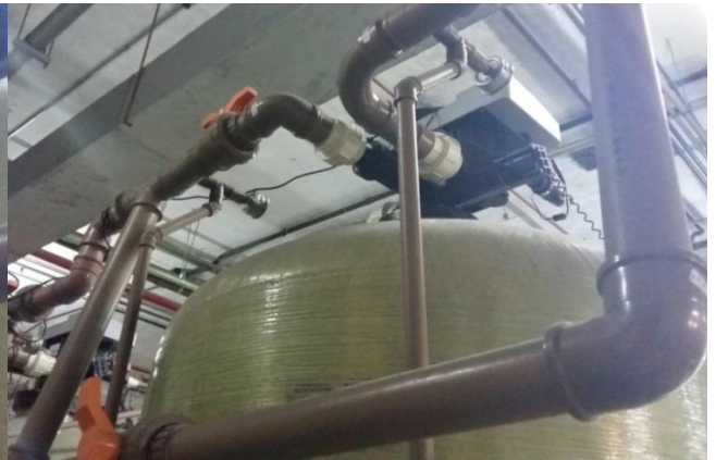
Figura 29 – By Pass da Planta Piloto
