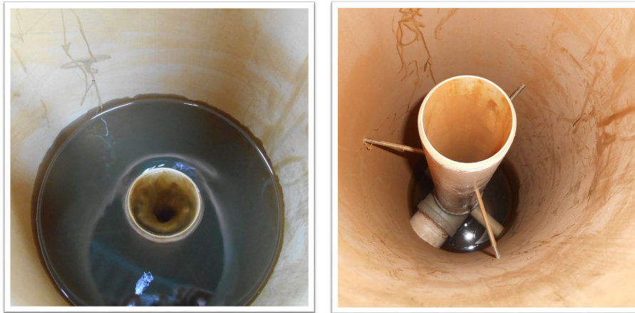
Figure 12 – Water collector inside the submerging structure providing a constant external pressure on the leak.
